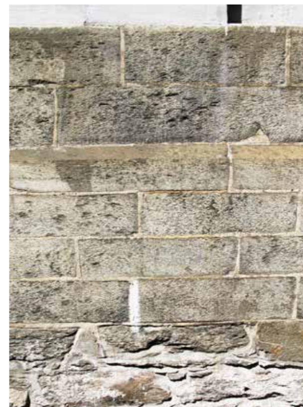
Fig 13. The lower wall of St. Paul's, detail from the exterior of the southern aisle, showing the rough foundations of natural stones (cf. fig. 7 and 9) upon which a c. 1 m. high socle of hewn stones with a simple chamfered moulding has been placed to carry the wall.
